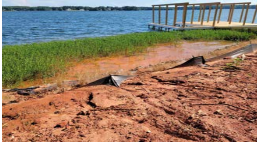
Failed silt fence along Lake Gaston Shoreline. Also notice the soil erosion tracks and muddy water along the shoreline.
